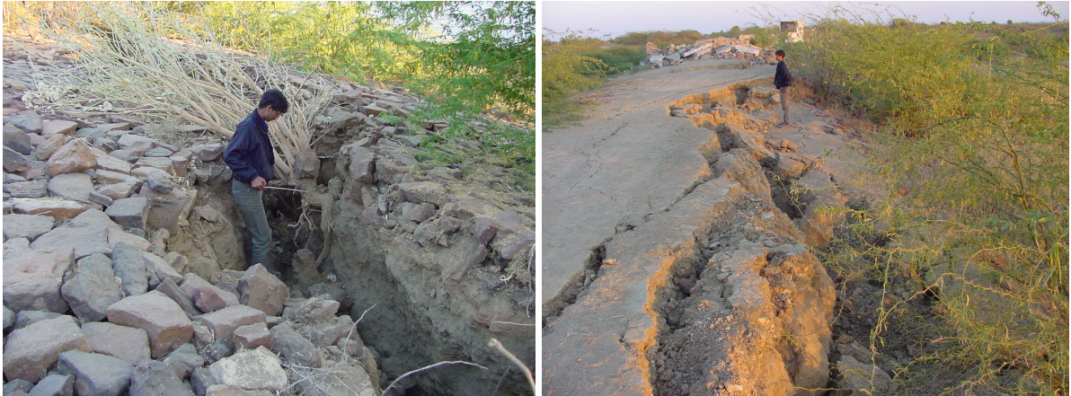
Fig. 3: Embankment dam damage caused by the 2001 Bhuj earthquake in India (about 245 damaged or deficient dams needed repair and seismic upgrading after the earthquake)
