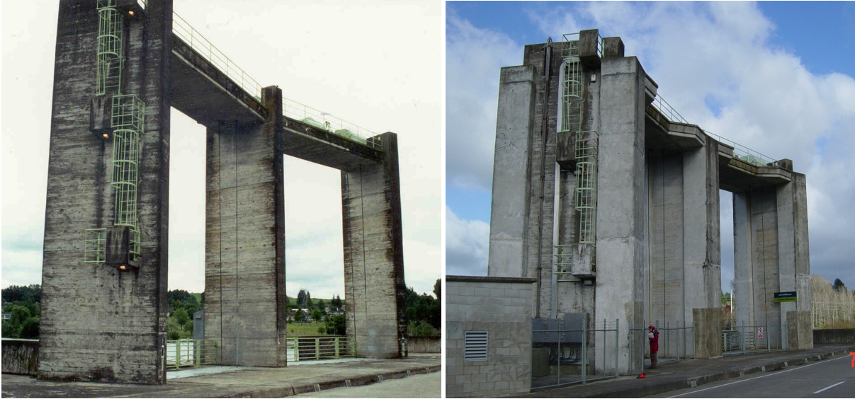
Fig. 2: Seismic strengthening of spillway gate structure located on the crest of the 56 m high Whakamura gravity dam in New Zealand (left: original design of 1956 based on pseudostatic acceleration of 0.1 g; right: strengthened structure with design acceleration of 1.9 g (Foster and Black, 2003).
