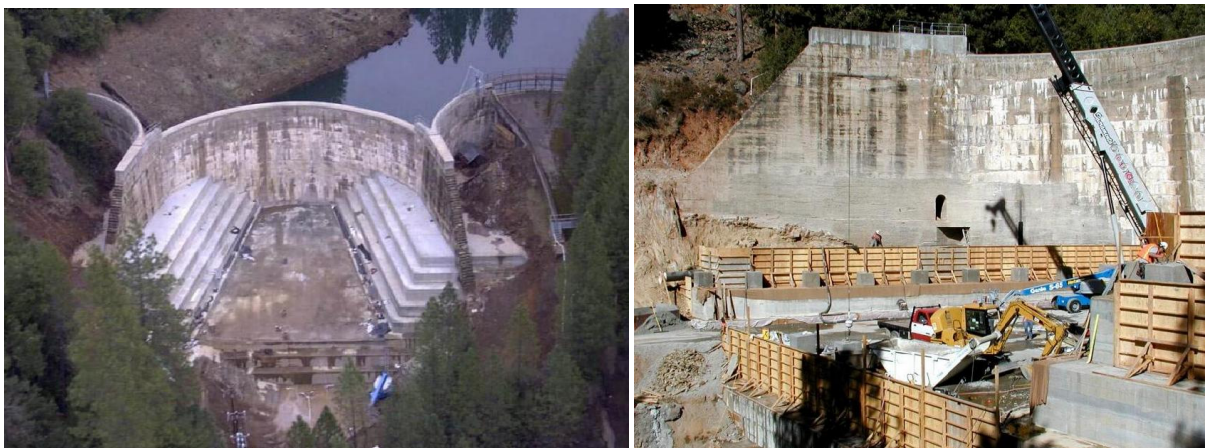
Fig. 8: Seismic strengthening of Weber multiple arch dam in California: strengthening of abutments by RCC block (left) final stage; (right) construction state (Photos D. Babbitt).
